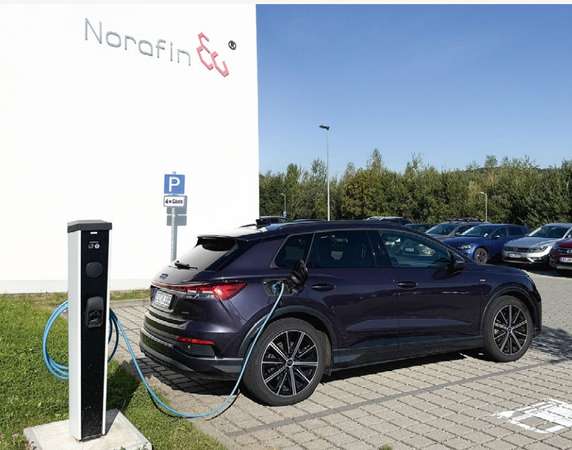
EV charging station, customer parking lot, Norafin Industries (Germany) GmbH
